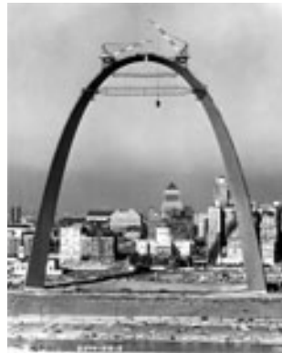
United States Jefferson National Expansion Memorial, St. Louis, Missouri, under construction, 1965 From the Collections of Arteaga Photos Ltd.
